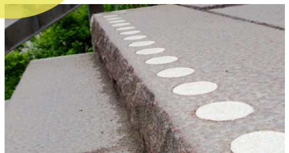
White sunken circle markings on the upper landing.
